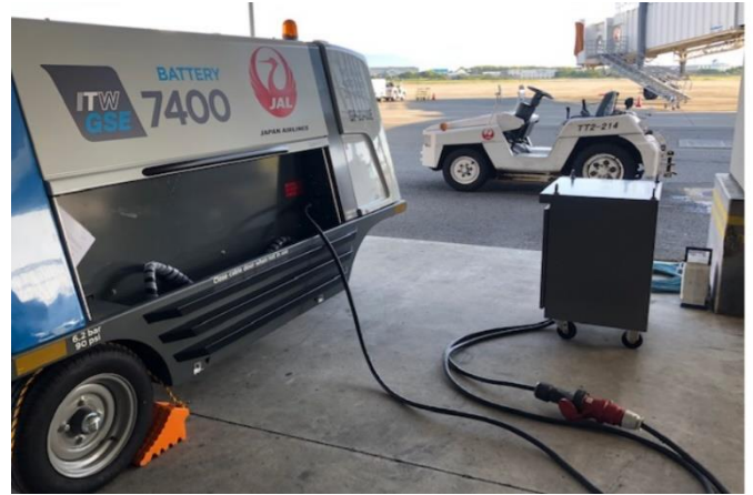
Converting the power plug used for the snowplow vehicle heater made it possible to install the charging infrastructure.
